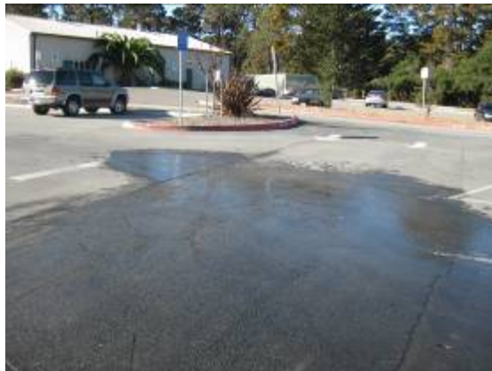
Water up-swell in Parking Lot C.
