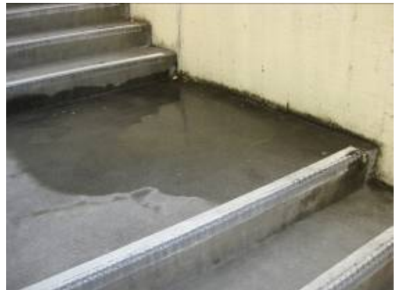
Standing water (w/algae) on stair landing of south-side of Physical Science Building
