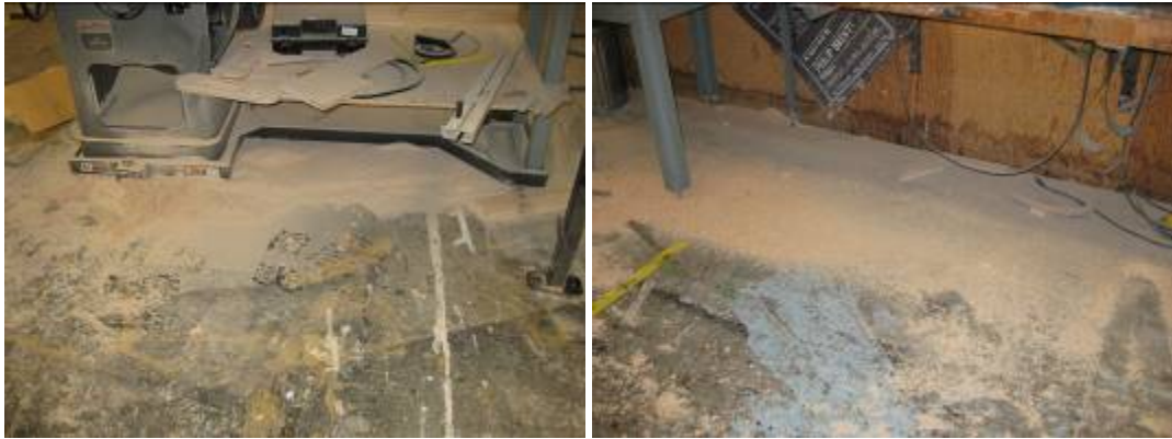
Accumulated sawdust from mill operation.
